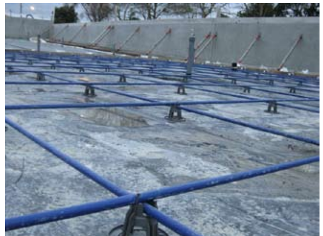
Layout of the strand at 800mm centres supported by concrete slab bar chairs, with a layer of polythene covering the underneath grade.
